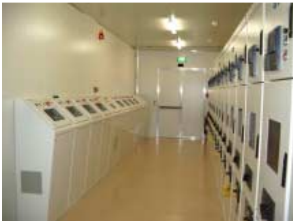
Left: The main control and switch room with the 11kV switchgear on the right and the desk type control panel with 8 IntelliSys and a Power Station Controller
